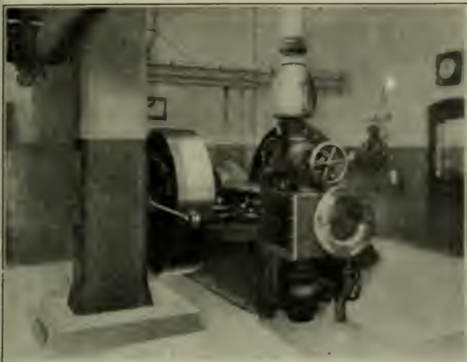
FIG. 9. SMALL GENERATING SET
